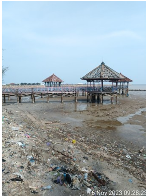
Figure 4. The condition of the pier, which is dilapidated and not maintained
